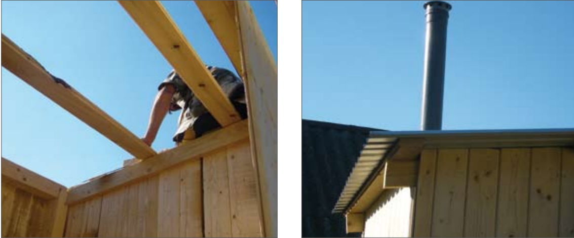
fig. 7: Construction of roof-bars from wood (left) and the roof-covering with zinc-covered metal-sheet (right)
