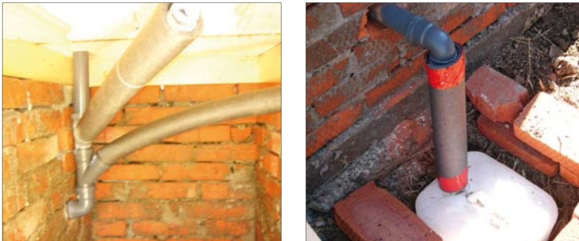
fig. 10: Urine hose 25mm with insulation and PP-pipes 50mm inside the faeces chambers (left); Small 20 litre urine container outside the toilet (right)
